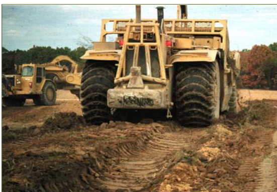
Compaction caused by twin-engine scrapers
